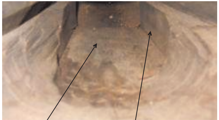
Inside view looking down: The Center Board (# 3) is chiseled down and rounded into a semi-circle until it reaches the next board (# 2) under it. The #2 board is not chiseled down any and is straight. Part of it is a stop and holds the pipe in place with shims. Also the #3 (Center Board), after it has been chiseled down on the sides into a semi-circle, is then cut straight back. The end stops the cone pipe at 1 & 3/4" before the end and the remainder of the board helps holds it in place with shims.
