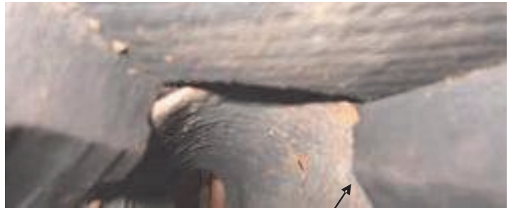
Inside view looking up: Note the three boards that are cut a little at 90 degrees 1 & 3/4" from the end. This is stop/hold the end of the cone pipe.
